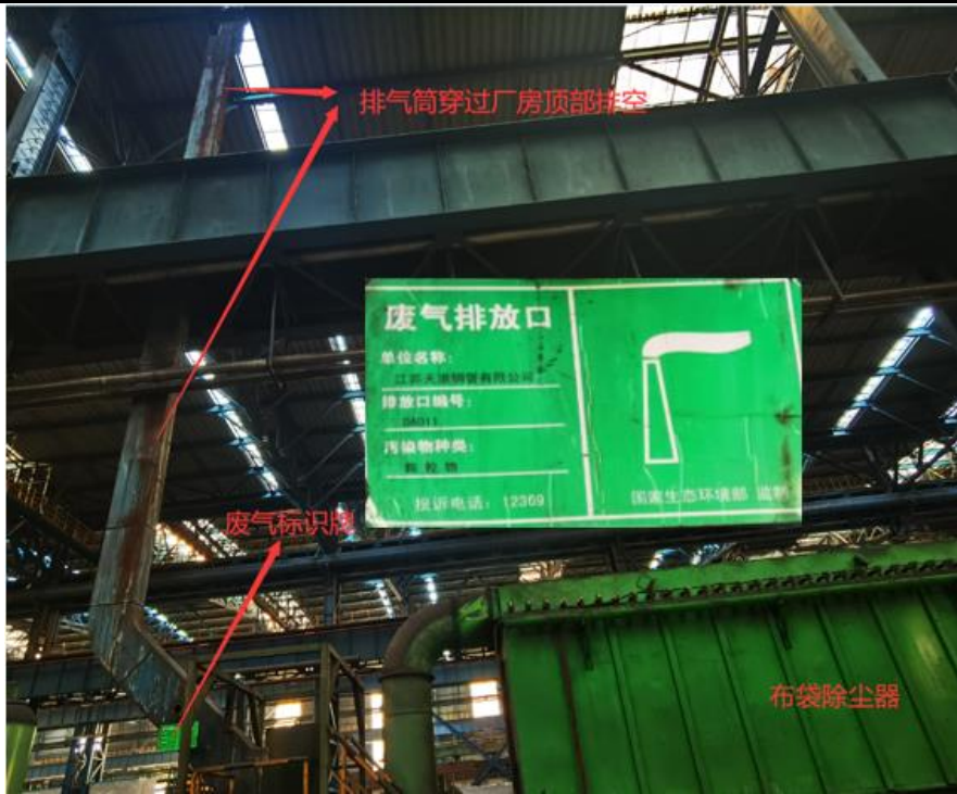
DA011 1#吹吸灰废气排放口及治理措施
